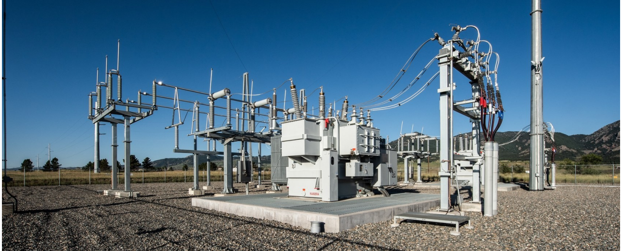
A distribution substation. Fixed sites are small enough to sit inside a single frame and repetitive enough that change between acquisitions, rather than any one image, carries the information.
